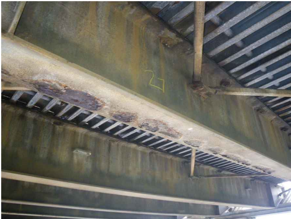
Photo 2: Span 2, Transom T27, Bottom Flange, Looking Northeast - Loss of galvanization and pitting section loss.
