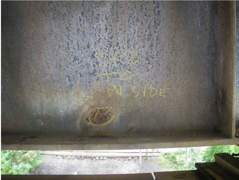
Photo 3: Span 3, Transom T0, Web, North Face, Looking South - Localized pitting section loss at area of failed galvanization.
