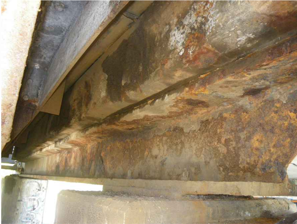
Photo 9: Span 9, at Pier 9, South Support Floorbeam, South Face, Looking Northwest - Section loss and pitting along full height.
