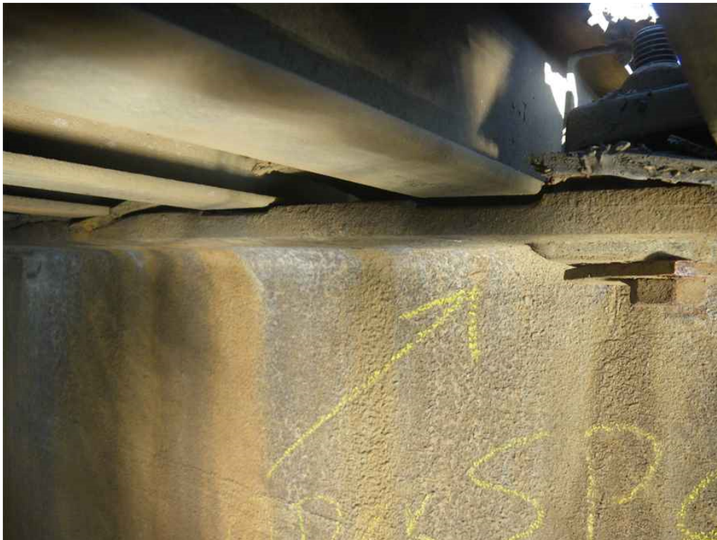
Photo 6: Span 6, Transom T12 Top Flange below 10th Roadway Deck Panel from East Curb, South Face of T12, Looking North - Four purlins have mutual wear with transom top flange, caused by loose panel above.
