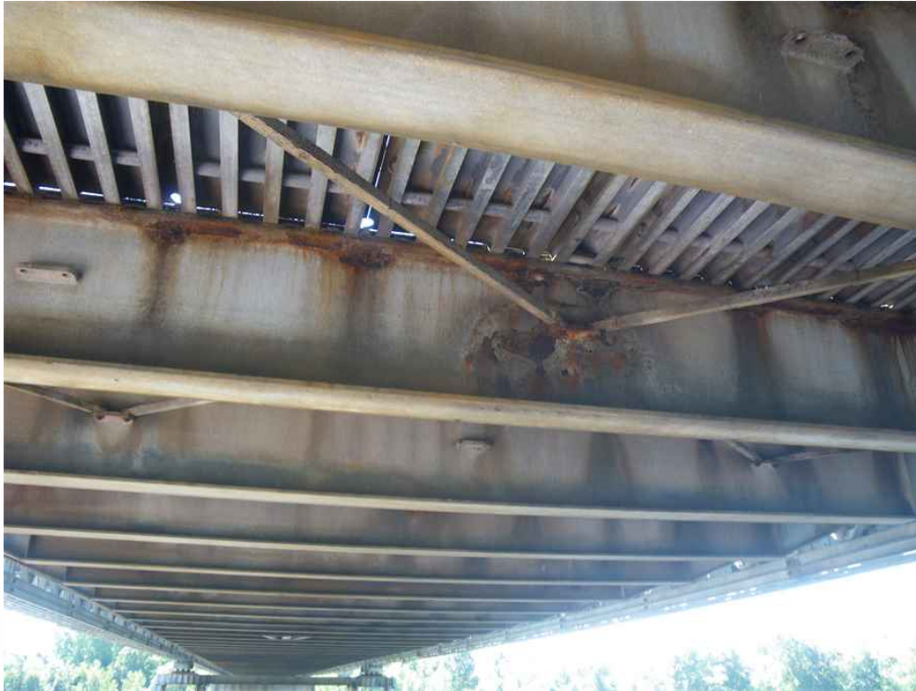
Photo 1: Span 7, Transoms in Northern Third of Span, Looking South - Areas of galvanization loss, and light to moderate surface rust at bottom of web.
