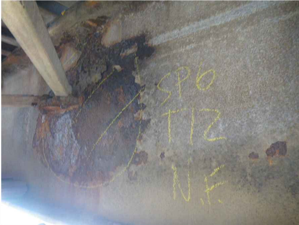
Photo 7: Span 6, Transom T12, at Midspan, Web, North Face, Looking Southeast - Up to 1/32" section loss on web around floor system bracing connection.
