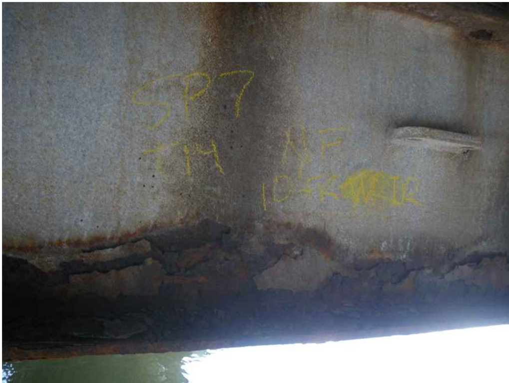
Photo 8: Span 7, Transom T14, 10'-0" from West Truss, Bottom Flange, North Face, Looking South - Up to 1/8" section loss at north edge of bottom flange.
