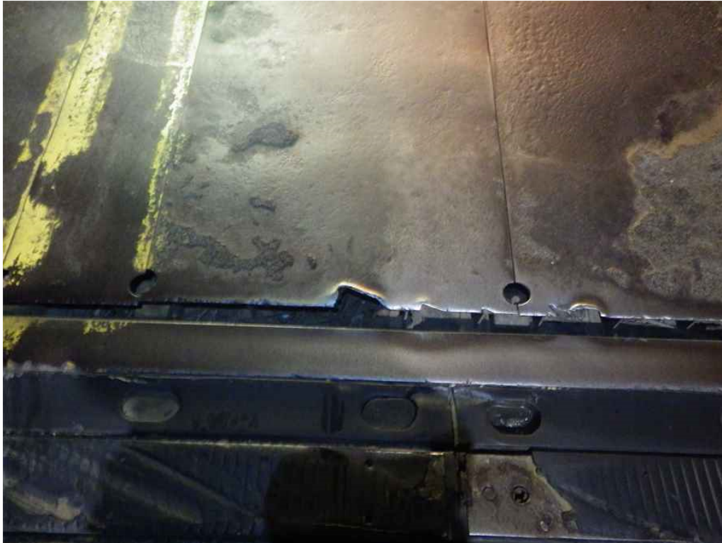
Photo 5: Span 2, Roadway Deck Panel South of T12, 11th Panel from East Curb, Looking North - 3" long by 4" wide fracture/100% section loss.
