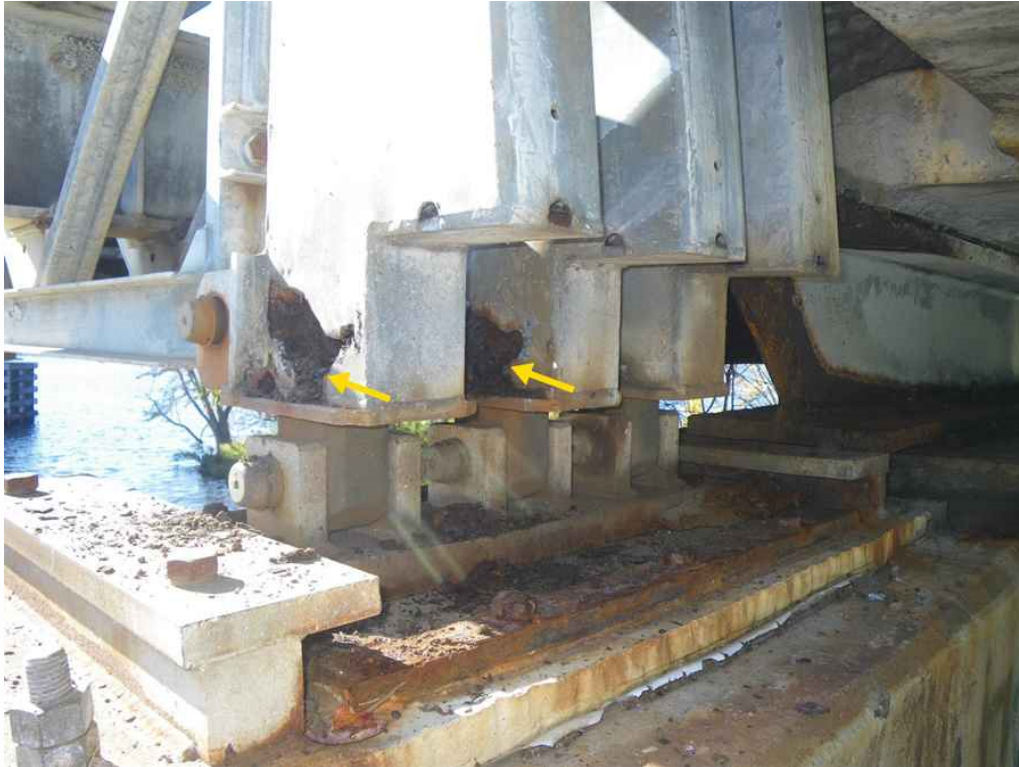
Photo 37: Span 8, East Truss, at Pier 8, East and Center End Posts, East Faces, Looking Southwest - Holes in east faces. Note north face of support floorbeam for span 9 reinforced concrete deck.
