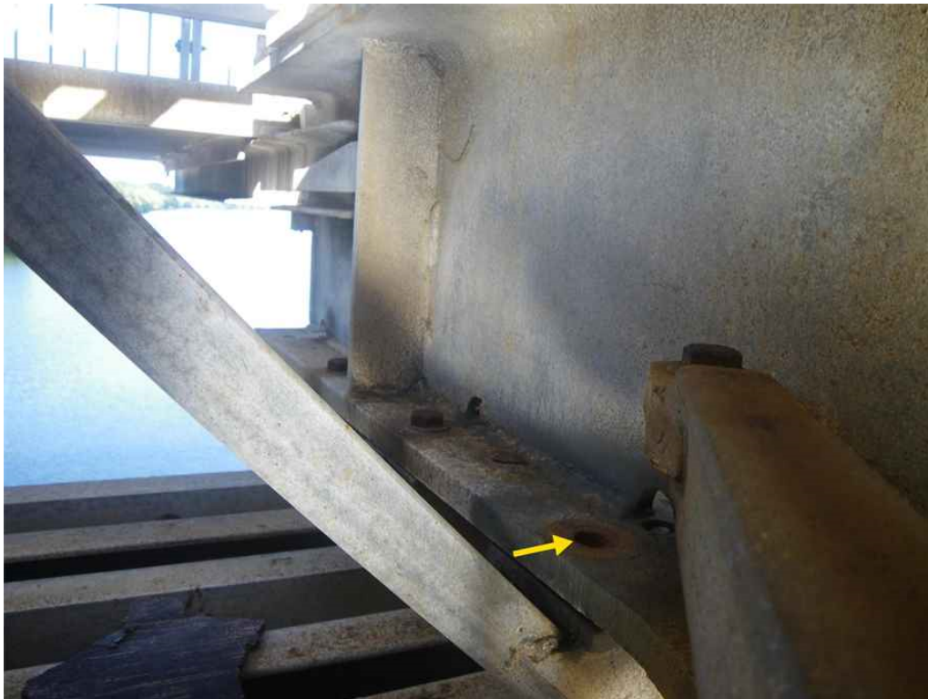
Photo 22: Span 3, Transom T16 at West Truss Bearing Area, Looking West - One bolt missing in southeast corner of transom bearing area. Note galvanization loss and surface rust on bolts.
