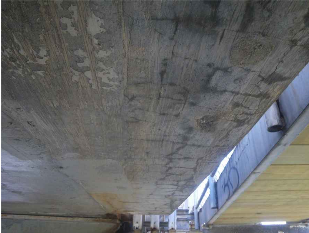
Photo 9: Span 9, Underside of Deck, At West Fascia, Looking South - Hairline map cracking with moisture throughout edge of deck. Note timber shielding in place below concrete sidewalk.
