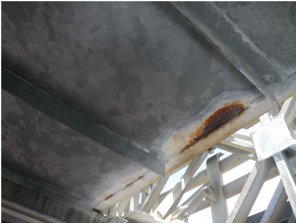
Photo 12: Span 5, Underside Sidewalk, Between T8-T9, Looking East - Moderate surface rust on underside of steel tread plate at edge.
