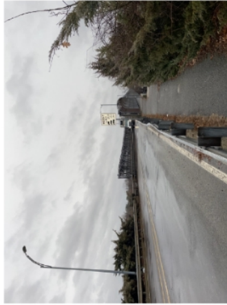
③ At bridge weight posting sign that reads: "20, 25, and 28 tons."
