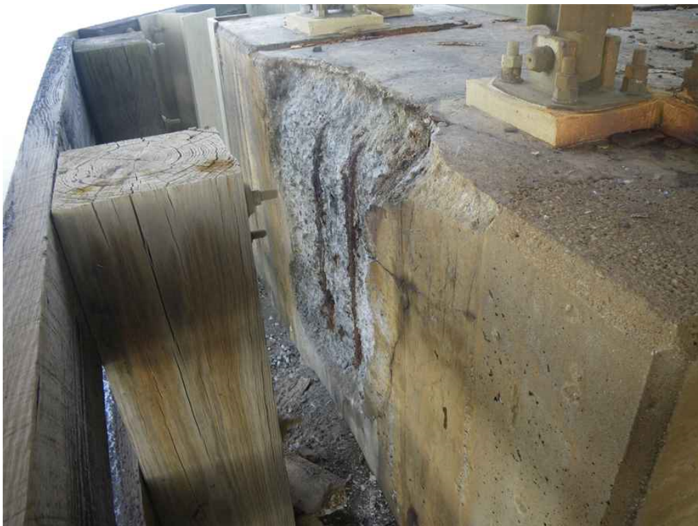
Photo 46: Pier 6, West Pedestal, South Face, Looking Northwest - Spall with exposed rebar and punky concrete.
