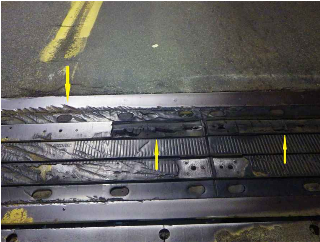
Photo 17: South Abut., Deck Joint, S.B. Lane, Lkg. South - Gouged & worn elastomeric cover exposing the internal plates w/ two missing sections of internal joint plates. Note gouging to joint armor angles.
