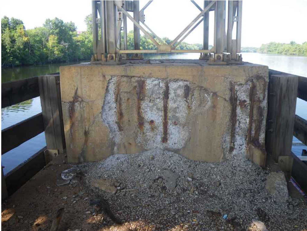
Photo 45: Pier 3, West Pedestal, East Face, Looking West - Spalls with exposed rebar with section loss.
