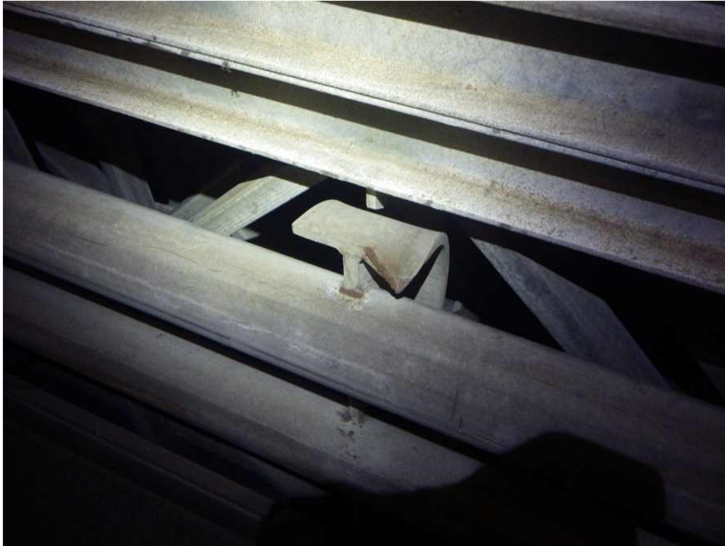
Photo 13: Span 8, West Rail Post at T9, Looking Southwest - Impact damage to north flange bent downwards.
