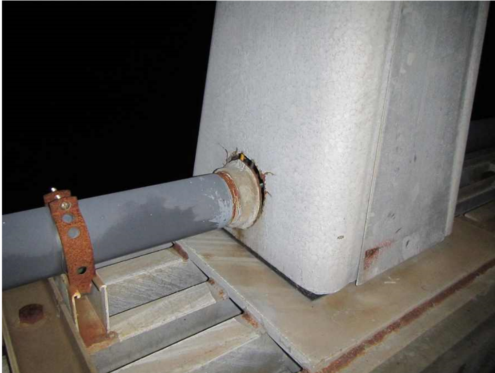
Photo 15: Span 5, Lighting Standard on East Truss, at South Third Point in Span (Pole Marking "20L"), Looking Southeast - 100% cracked weld for conduit connection, w/ cracks emanating east and west.
