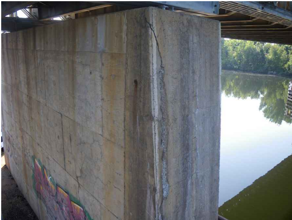
Photo 48: Pier 4, Pierwall, North and West Faces, Looking Southeast - Hairline map cracking with moisture on N face, and hairline map cracking with efflorescence and spall within hollow area at NW corner of W face.
