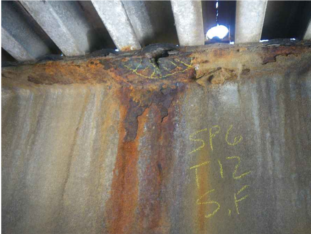
Photo 23: Span 6, Transom T12, 8'-0" from East Truss, Top Flange, South Face, Looking North - Hole at edge of top flange, surrounded by area of section loss.
