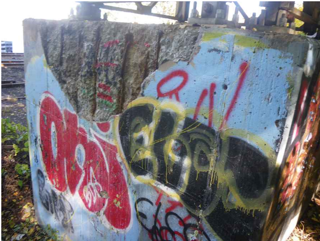
Photo 44: Pier 1, West Pedestal, West Face, Looking Northeast - Spall with exposed rebar with heavy surface rust and corrosion.
