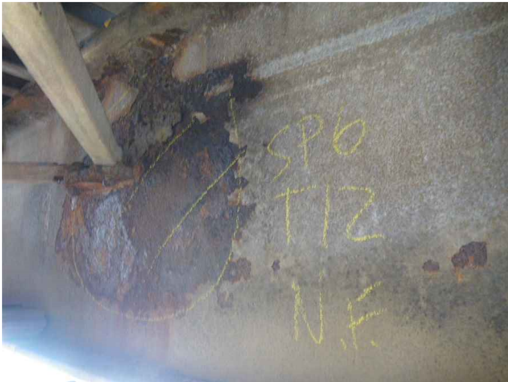
Photo 24: Span 6, Transom T12, at Midspan, Web, North Face, Looking Southeast - Up to 1/32" section loss on web around floor system bracing connection.
