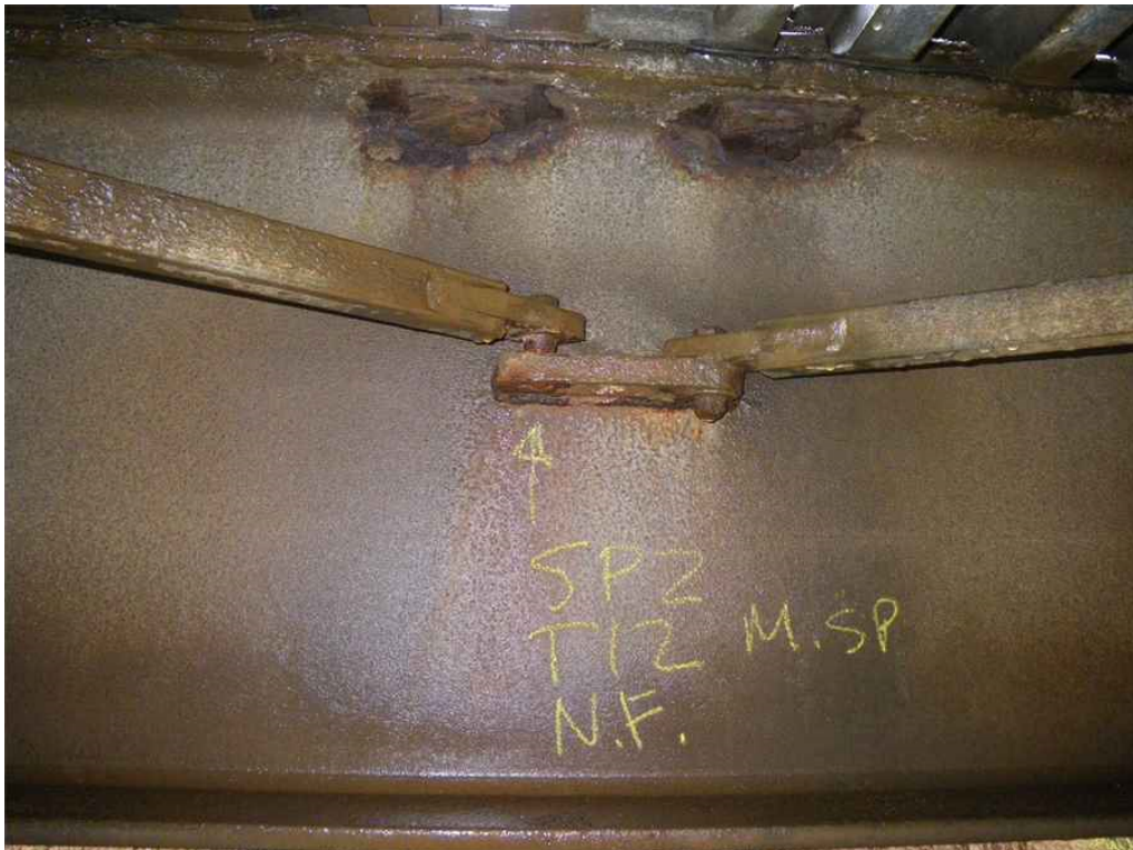
Photo 26: Span 2, Floor System Brace Between T12-T13, Connection at T12 for Middle East Brace, North Face, Looking South - Loose/disengaged bolt at bracing member connection.
