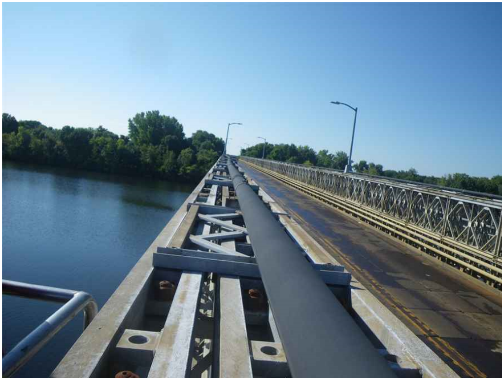
Photo 16: Span 6, Conduit on East Truss, Looking South - Conduit throughout span not seated on the steel brackets, and conduit has shifted.
