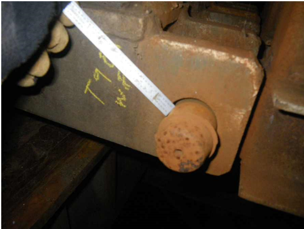
Photo 32: Span 1, East Truss, Lower Chord, West Lower Pin Between T9-Bearing, West Face, Looking Northeast - Loose pin with abrasion dust and up to 1/4" gap.
