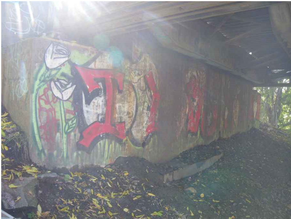
Photo 42: South Abutment, Breastwall and Footing, Looking Southwest - Graffiti on breastwall, and exposed footing.
