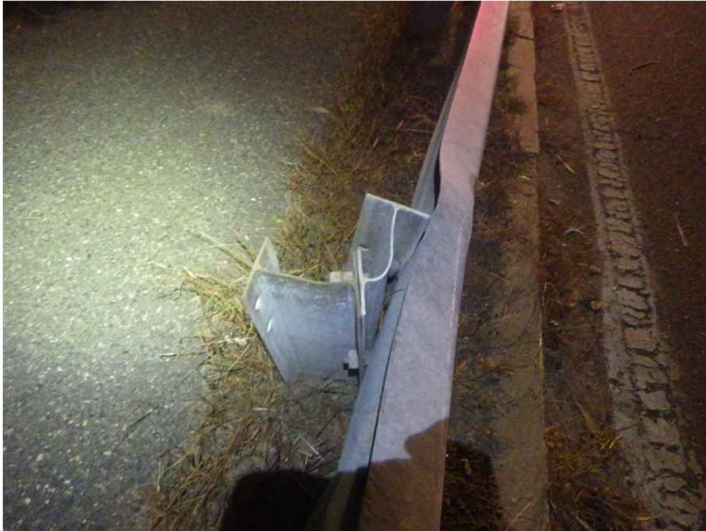
Photo 53: Northwest Approach Guardrail, Rail Post #11, Looking North - Collision damage to guardrail, and bent rail post.
