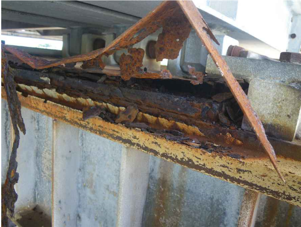
Photo 39: Pier 5, West Truss Bearing, Guide Plate, Looking Southeast - Failed galvanization with surface rust. Note sheet metal bearing cover section loss/holes and deterioration.
