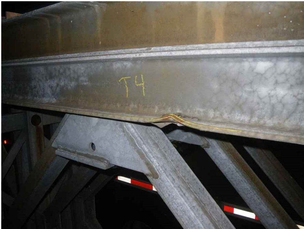
Photo 30: Span 2, East Truss, Upper Chord, East Bottom Channel located North of Pin Between T3-T4, East Face, Looking Southwest - East bottom flange bent upward.
