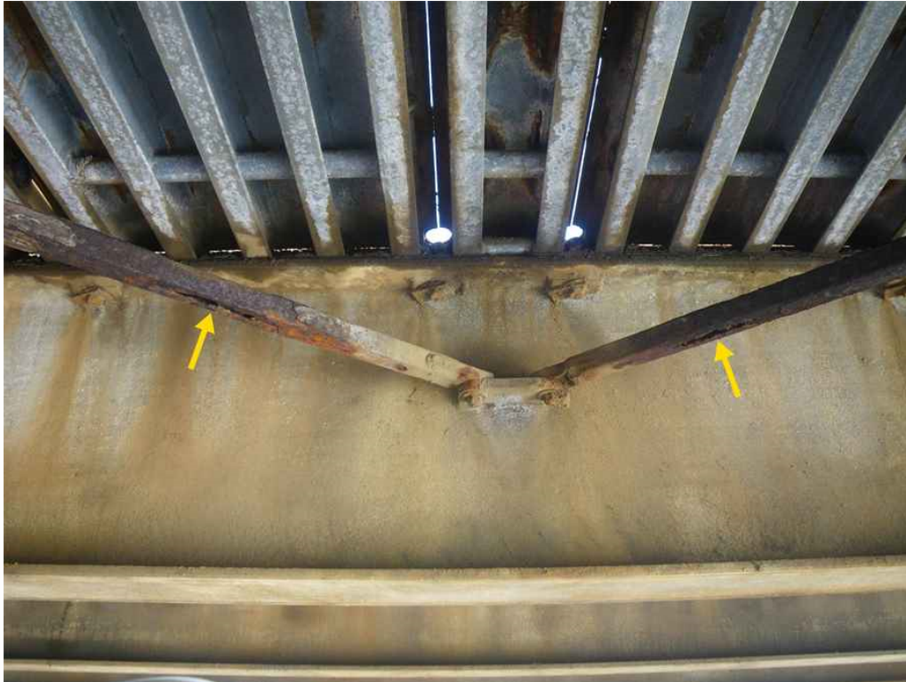
Photo 27: Span 4, Floor System Braces Between T17-T18, Middle East and West Braces Near T18, South Face, Looking North - Areas of up to 100% section loss.
