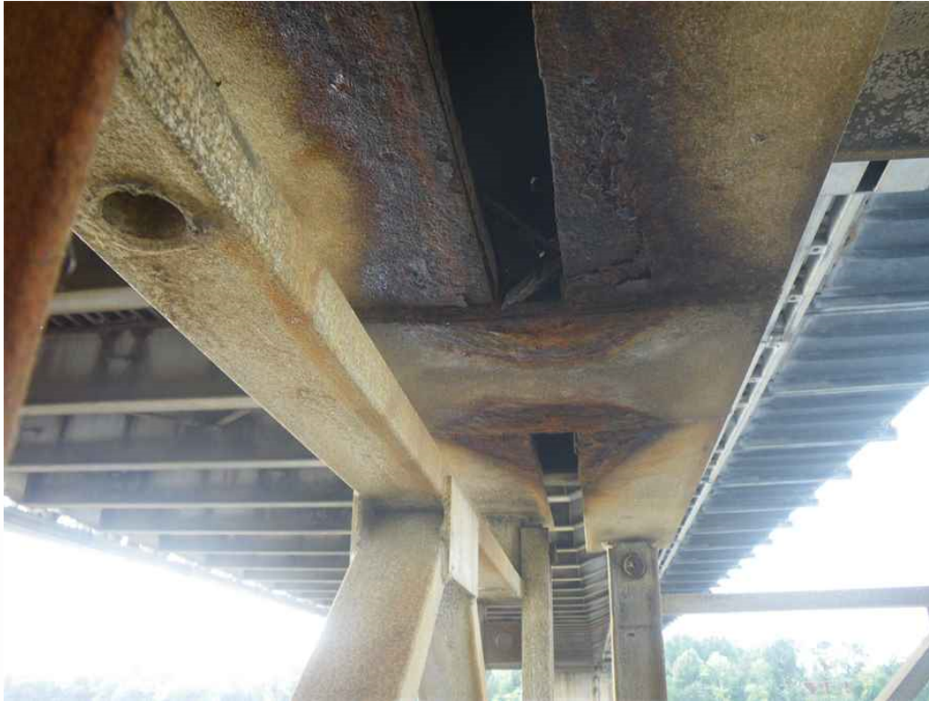
Photo 49: Pier 6, West Acrow Tower, East and West Distribution Beams, Underside, Looking South - Section loss on bottom flange of west distribution beam, along interior face of beam.
