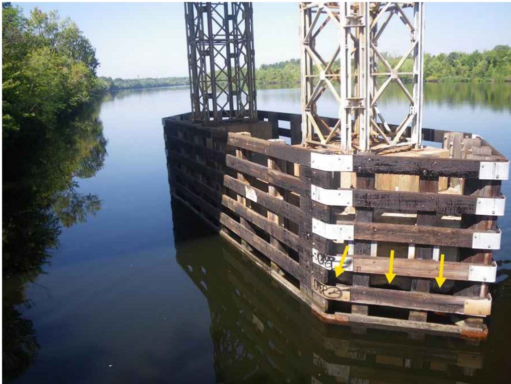
Photo 50: Pier 2, Pile Cap, South Elevation at East End, Looking Northwest - Spalls around base of pile cap.
