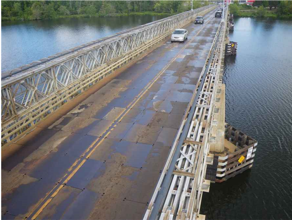
Photo 1: Span 4, Roadway Deck Panels, Looking North - General view of areas of missing epoxy aggregate wearing surface exposing surfaces of steel panels below.
