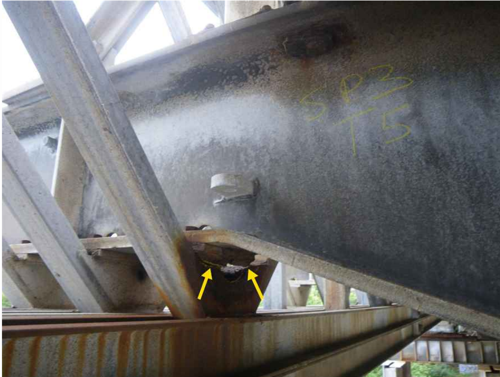
Photo 33: Span 3, East Truss, Lower Chord, Transom T5 West Panel Point Connection Plate, W Face, Lkg SE - Hole w/ adj full length crack of conn PL resulting in full separation on both sides of panel point.
