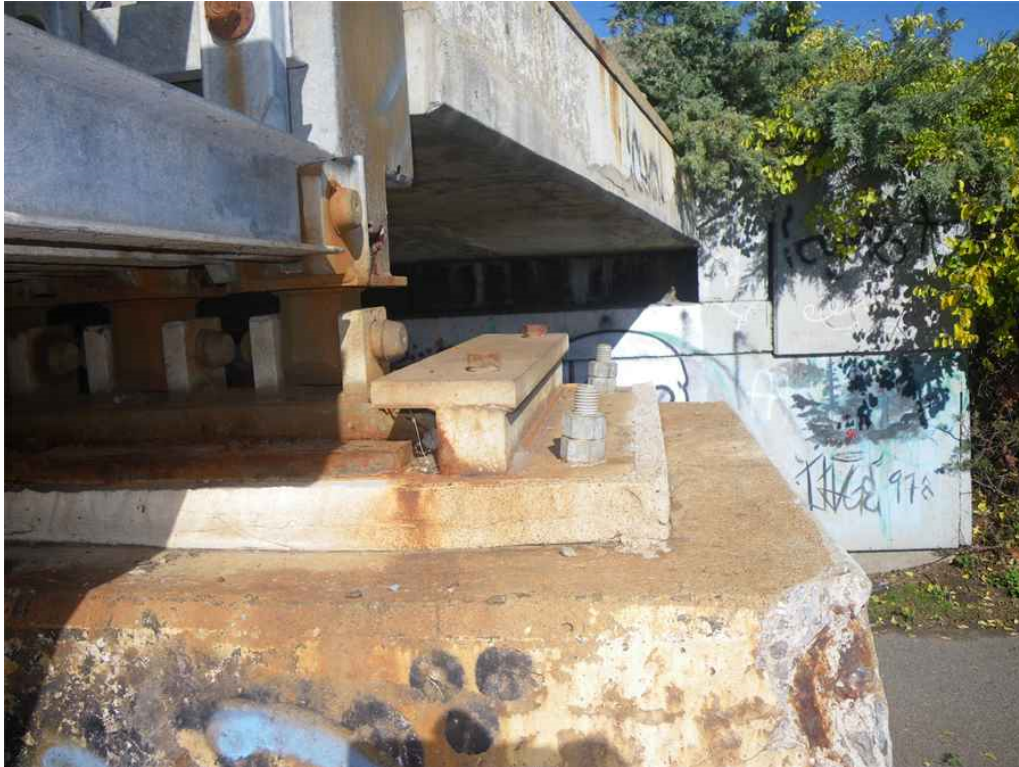
Photo 41: Pier 8, East Truss Bearing, East Anchor Bolts, Looking North - Anchor bolts bent to east. Note north abutment backwall with efflorescence, and graffiti on breastwall.
