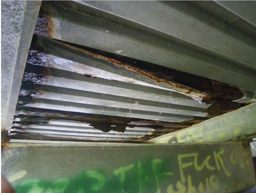
Photo 11: South Approach, SIP Forms under Sidewalk, near South Abutment, Looking Northeast - Areas of heavy rust and corrosion holes along SIP joints and edges.
