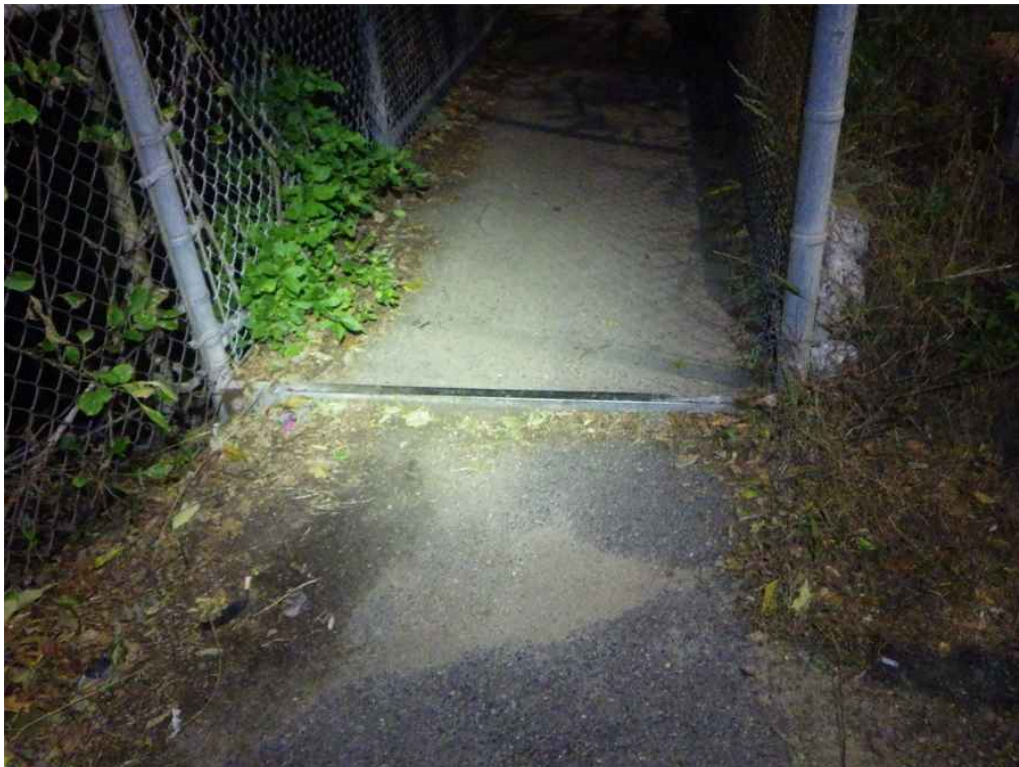
Photo 18: South Approach, Sidewalk, Looking North - Settlement throughout bituminous sidewalk with low points filled with debris.
