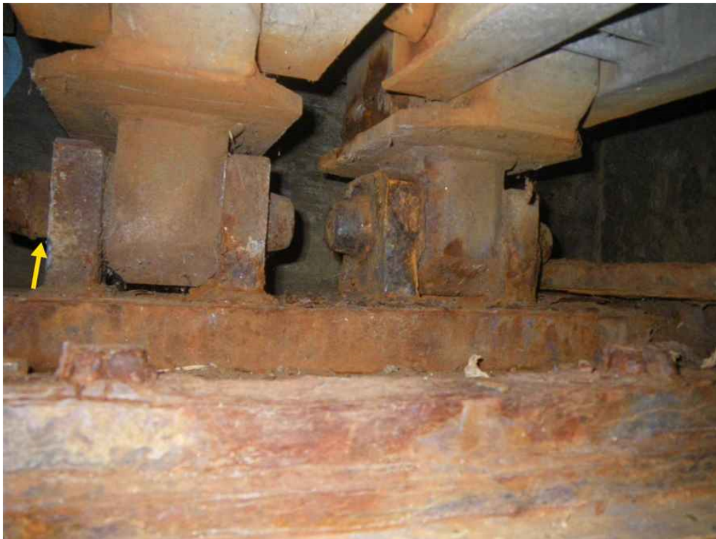
Photo 38: Span 1, East Truss, at South Abutment, West End Post, East Face, Looking Southwest - Pin and connection plate have heavy surface rust, and pin is missing retainer clip.
