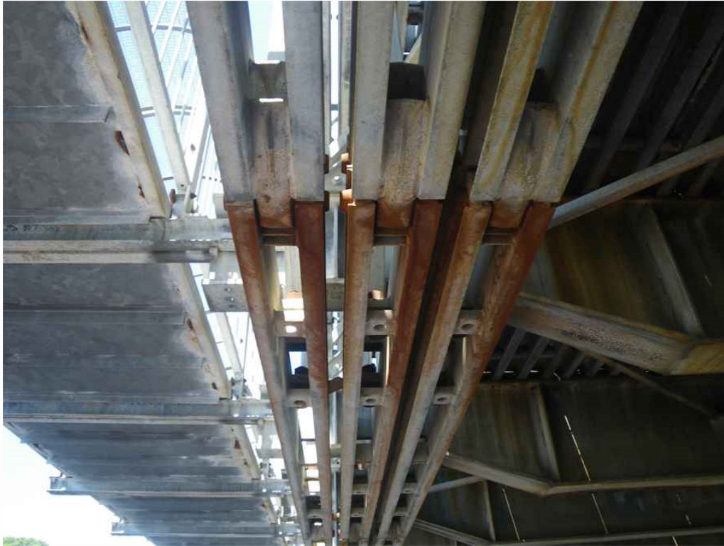
Photo 31: Span 7, West Truss, Lower Chord, All Lower Pins Between T5-T6, Underside, Looking North - All lower pins loose with abrasion dust.
