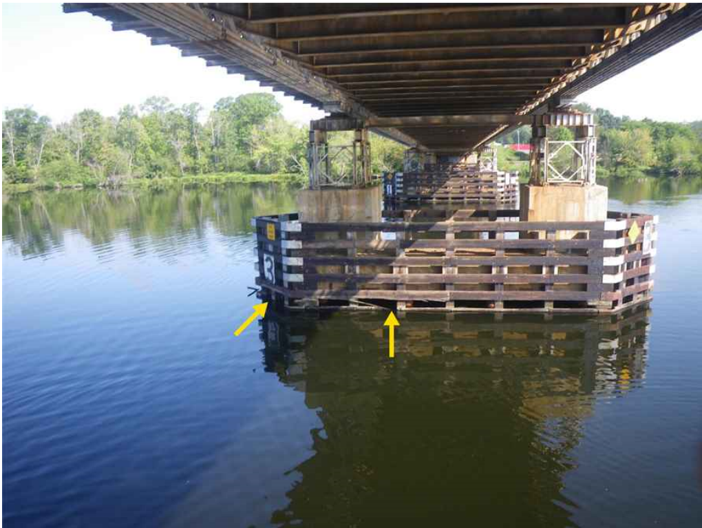
Photo 52: Pier 5, Timber Fender System, South Elevation, Looking North - Damaged waler 6th from top on west half of south face, and missing waler 6th from top at the west nose.
