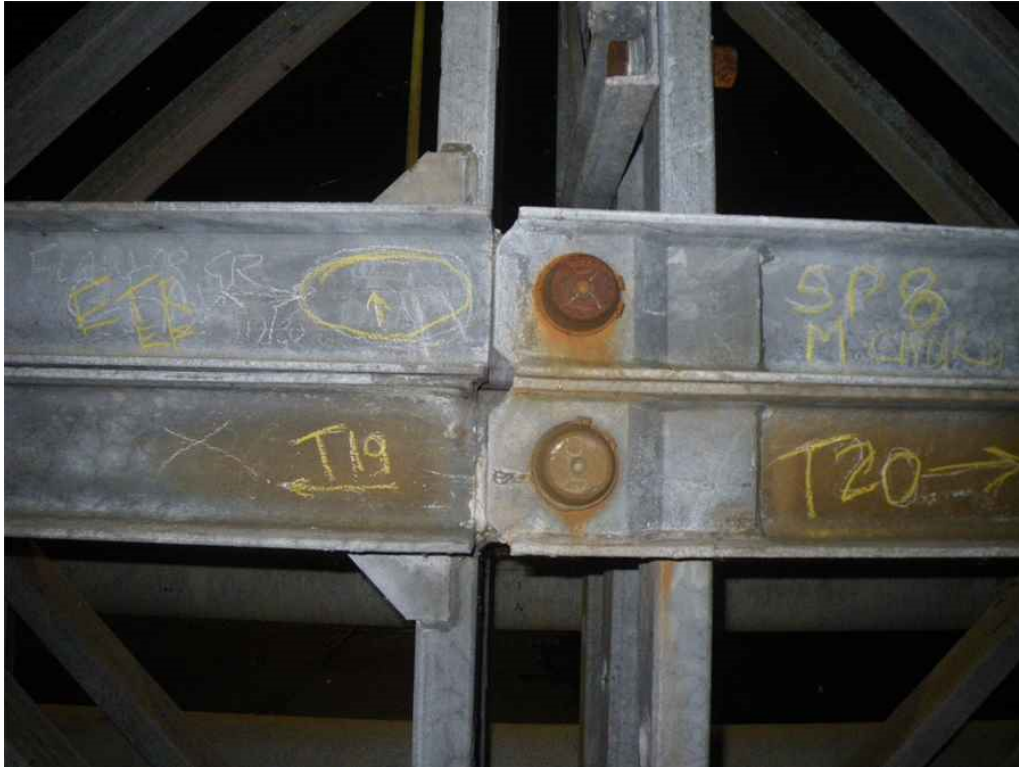
Photo 35: Span 8, East Truss, Middle Chord South of T19-T20 Pin, Upper East Channel Web, East Face, Looking West - Longitudinal flaw in channel web.
