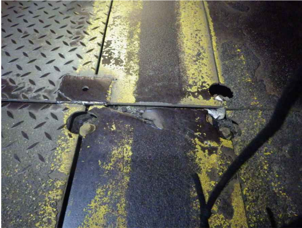
Photo 7: Span 5, Roadway Deck Panel South of T16, 6th Panel (Middle Panel) from East Curb, Looking North - Gouge at corner.
