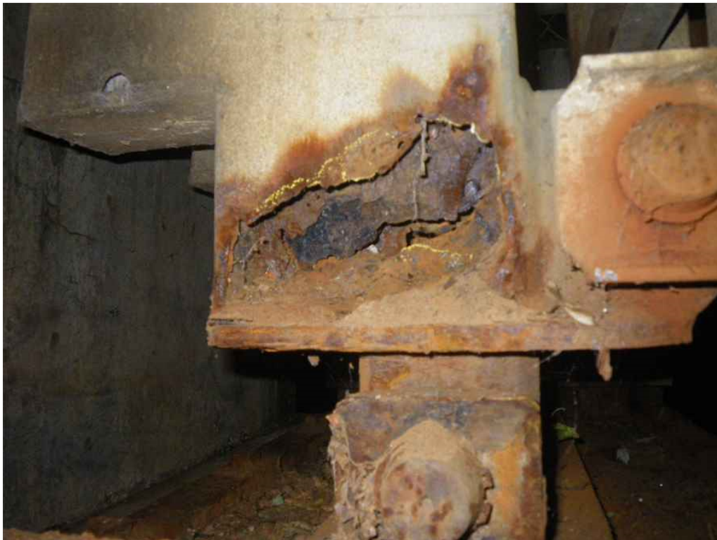
Photo 36: Span 1, West Truss, at South Abutment, East End Post, East Face, Looking West - Holes in east and west faces.
