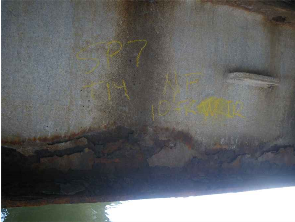
Photo 25: Span 7, Transom T14, 10'-0" from West Truss, Bottom Flange, North Face, Looking South - Up to 1/8" section loss at north edge of bottom flange.
