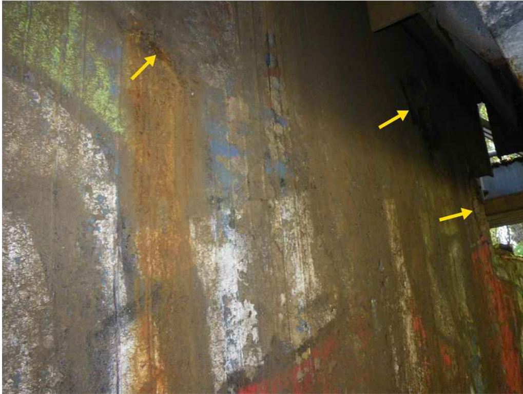
Photo 43: South Abutment, Breastwall, West Half, Looking Southwest - Three spalls with exposed rebar.
