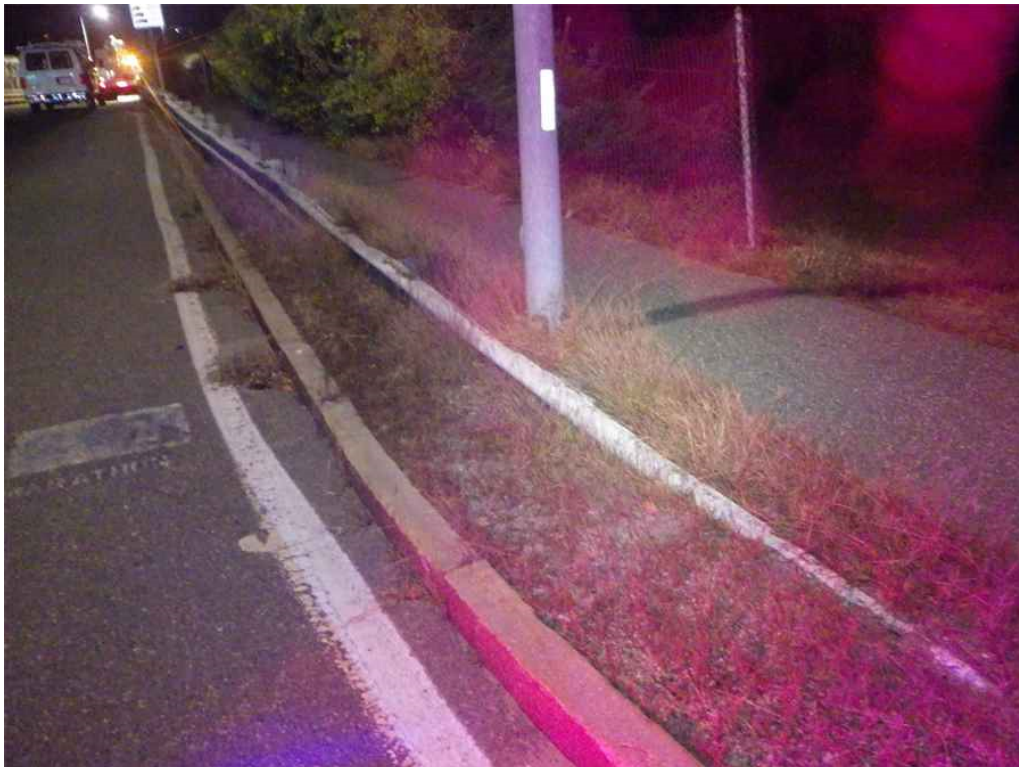
Photo 54: Northwest Approach Guardrail, Terminal End, Looking Southwest - Terminal end is buried and damaged.
