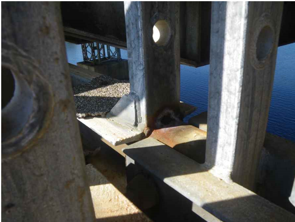
Photo 34: Span 6, East Truss, South of Pin Between T9-T10, West Vertical Member At Lower Chord Connection, North Face, Looking Southwest - Active corrosion at bottom of vertical member.
