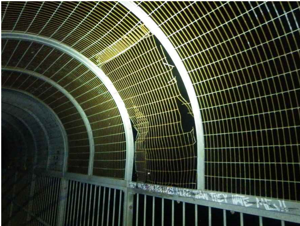
Photo 14: Span 4, Anti-Missile Fence on Sidewalk, between T8-T9, Looking Southwest - West half of previous repair on the anti-missile fence is torn and loose.
