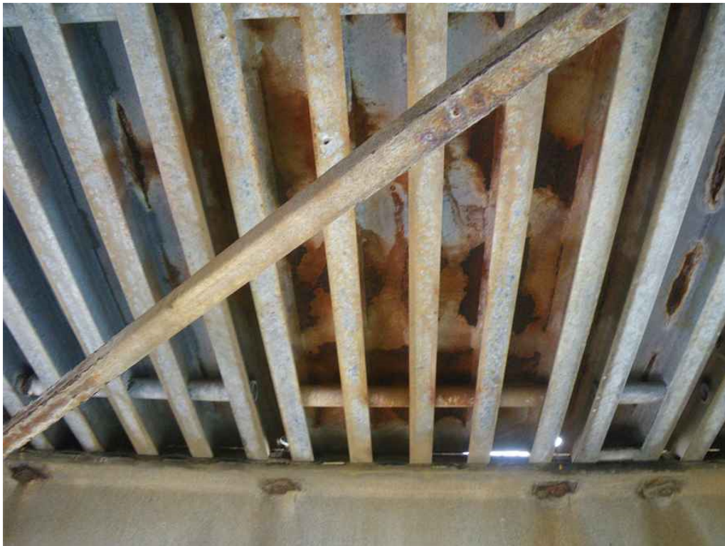
Photo 4: Span 4, Roadway Deck Panel between T4 and T5, 5th Panel from East Curb, Looking South - Failed galvanization and heavy surface rust on underside.
