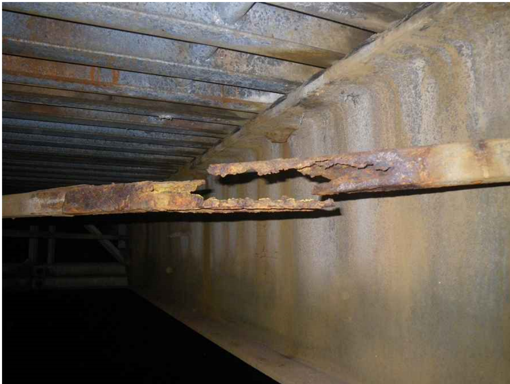
Photo 28: Span 2, Floor System Brace Between T7-T8, Middle West Brace near T8, South Face, Looking Northwest - Areas of up to 100% section loss.
