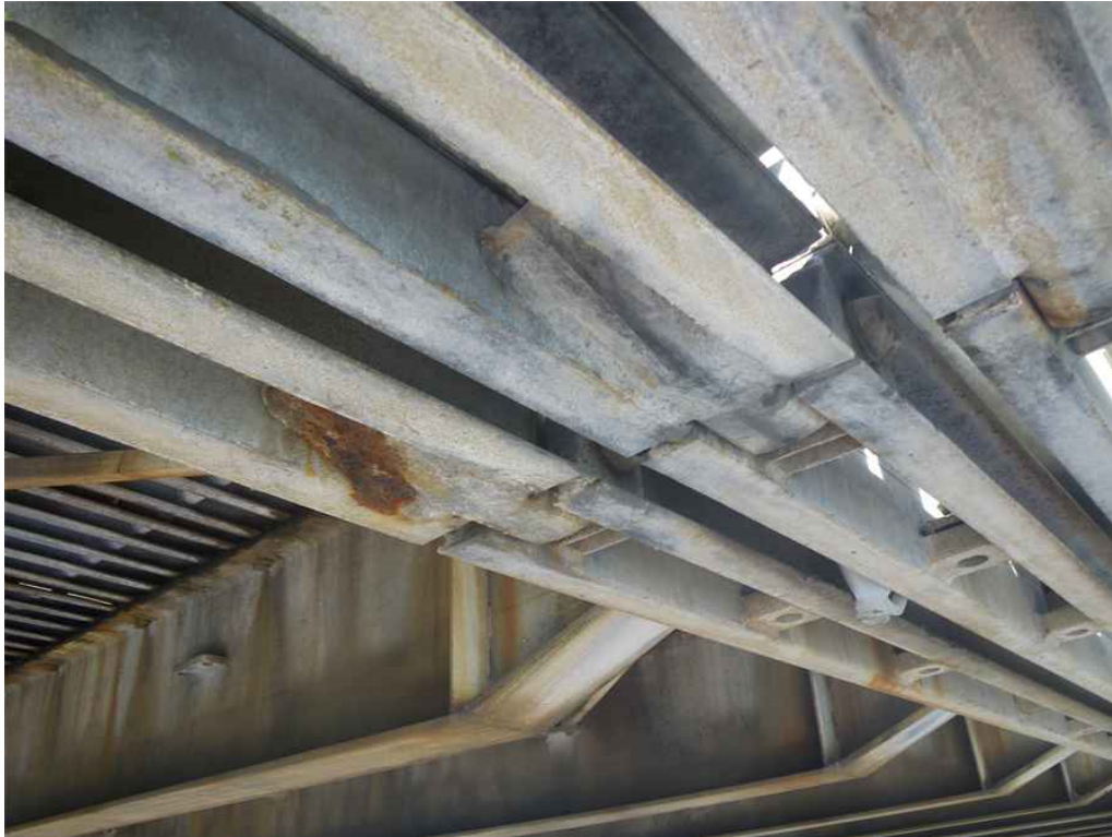
Photo 29: Span 4, East Truss, Lower Chord, Pin Between T17-T18, Underside, Looking Northwest - Loss of galvanization and surface rust.
