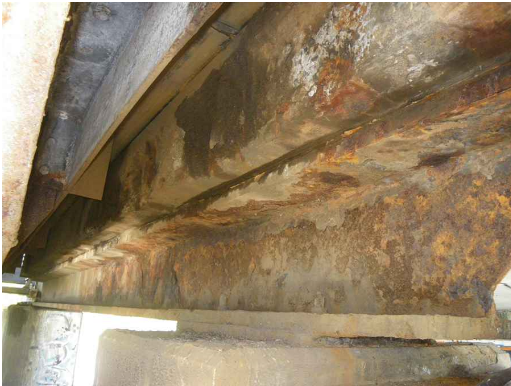
Photo 10: Span 9, at Pier 9, South End Conc Deck, and South Support Floorbeam, South Face, Looking Northwest - Spall with exposed reinforcing. Note floorbeam w/ section loss & pitting along full height.
