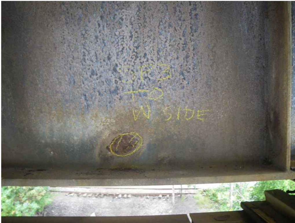
Photo 21: Span 3, Transom T0, Web, North Face, Looking South - Localized pitting section loss at area of failed galvanization.
