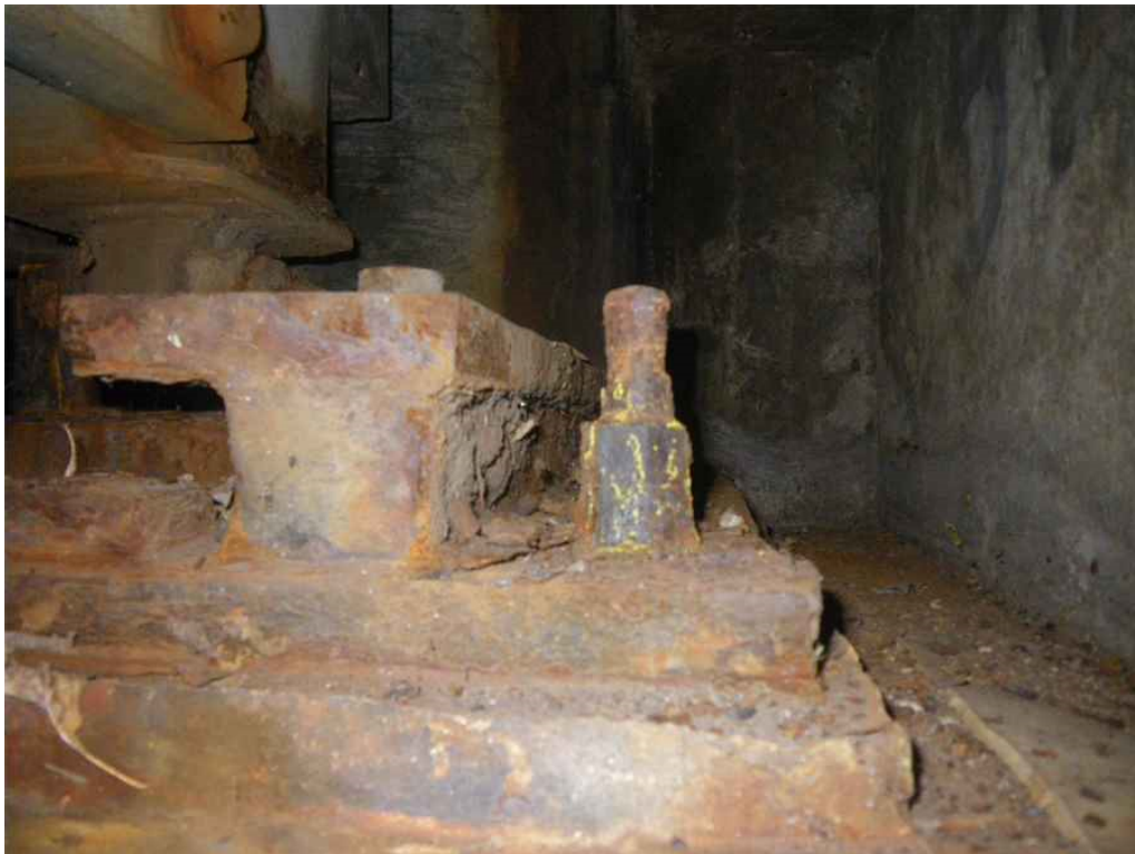
Photo 40: South Abutment, East Truss Bearing, West Anchor Bolts, Looking South - Section loss on northwest anchor bolt nut.
